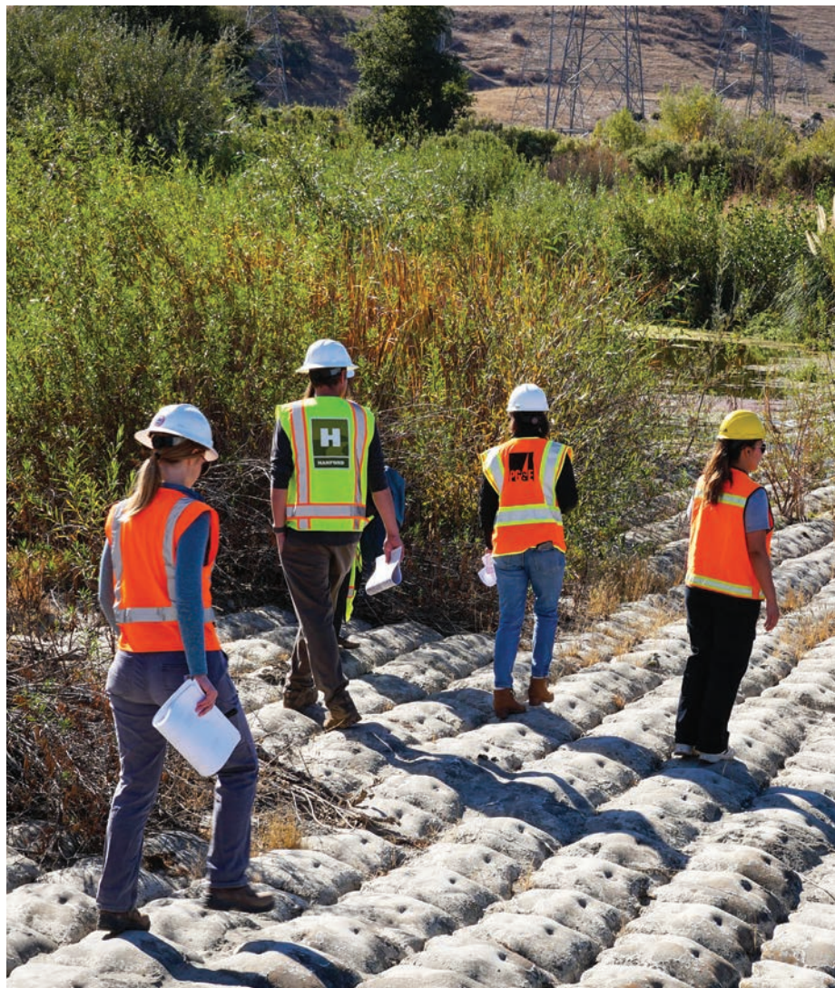
Officials inspect the PG&E gas pipeline protective apron over Alameda Creek near Sunol. Photo by California Trout
